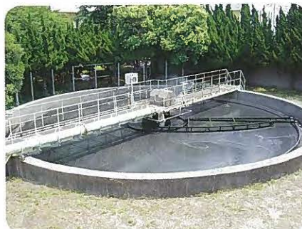
⑧汚泥濃縮槽
